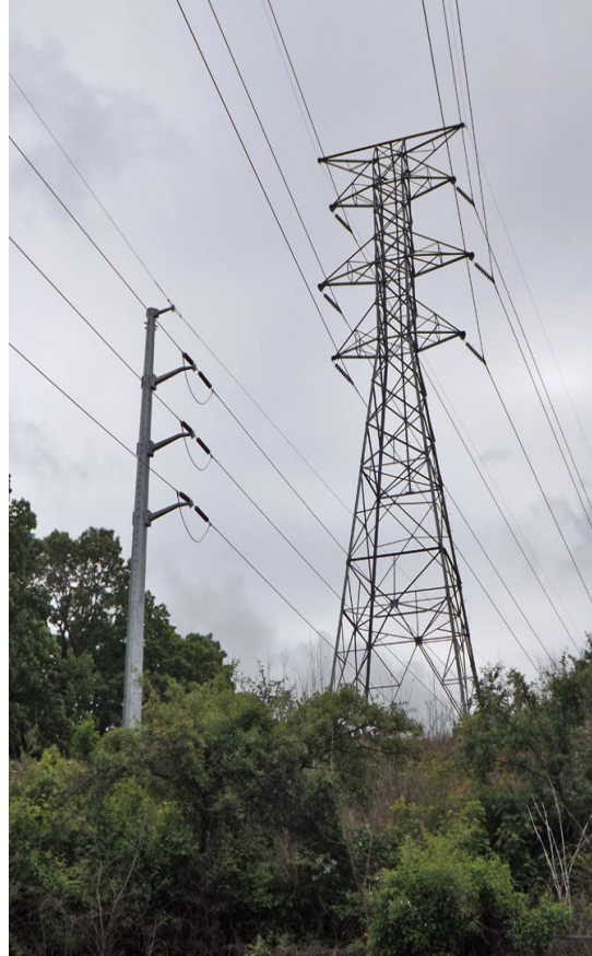
Electric Transmission Lines
